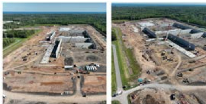
fairlife plant construction as of August 6th, 2024, Webster, NY. Photo credit: fairlife®
